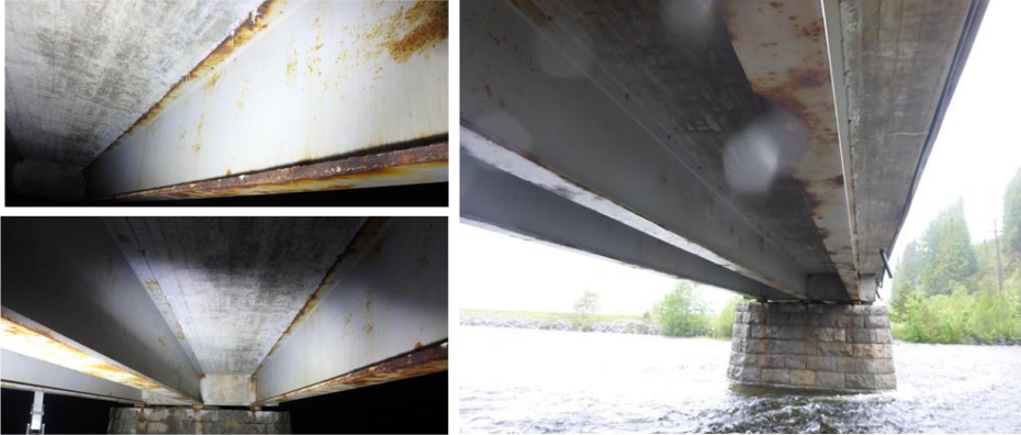
Figure 4. Bridge girders with corrosion
